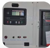
Control Panel & MCB
